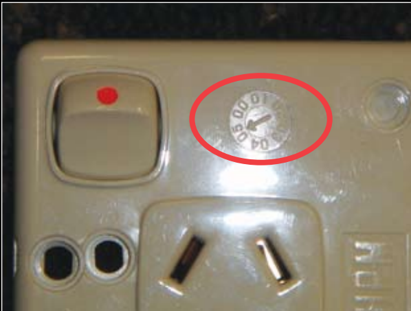
Fig. 2. Unapproved look-alike with close up of clock face. If the clock arrow points to '05' as in this photograph, the socket outlet may be unapproved.
